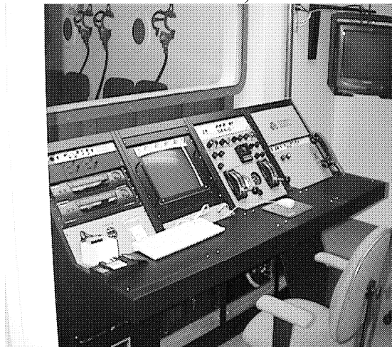
(Control Console with manual and computer controls)
